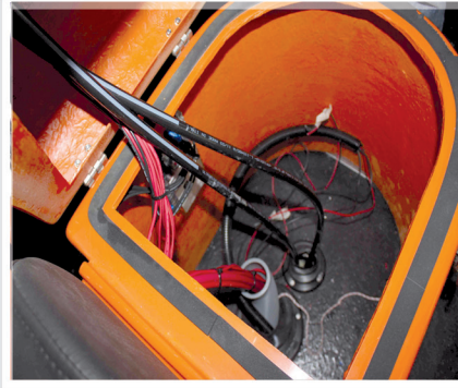
PIPE FOR ENGINE WIRES (INSIDE OF CONSOLE)
